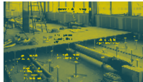
(Facing page and above left) DIGITAL WEAVE: SFMoMA Installation from Prof. L. Iwamoto Graduate Seminars & Studio: CAD/CAM TRANSLATIONS (Above) Underfloor Air Distribution Design Guide by Fred S. Bauman
